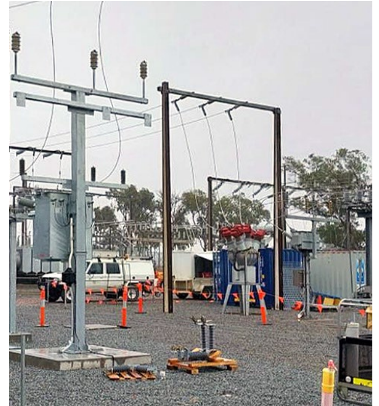
Upgraded Cleve Substation
