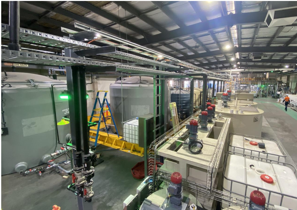
Figure 1. Renascor's PSG Demonstration Facility
