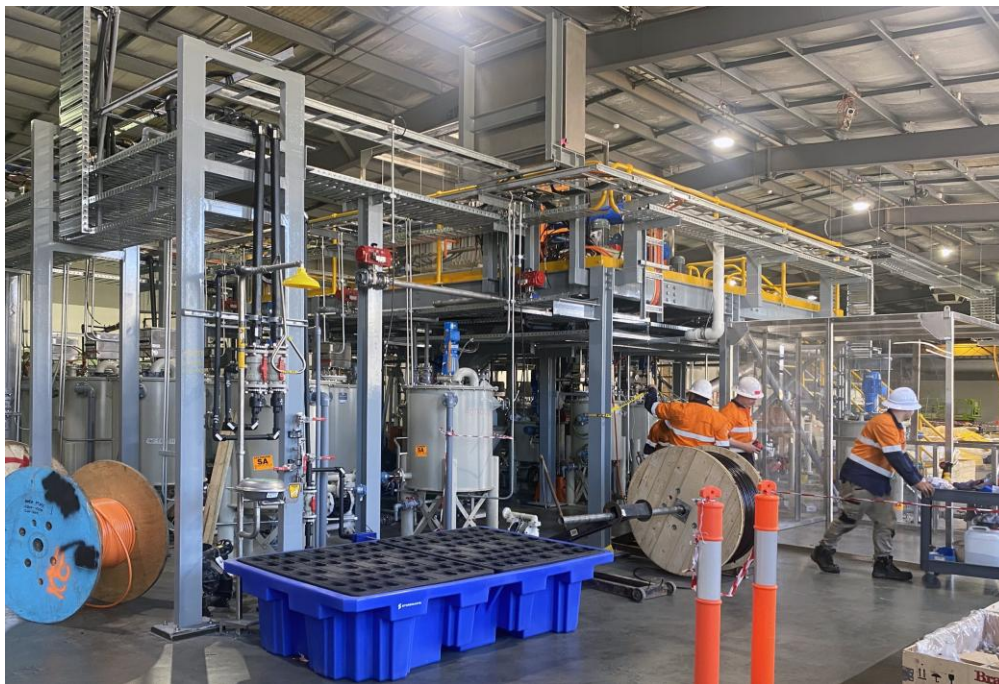
Figure 2. Processing equipment at the PSG demonstration facility
