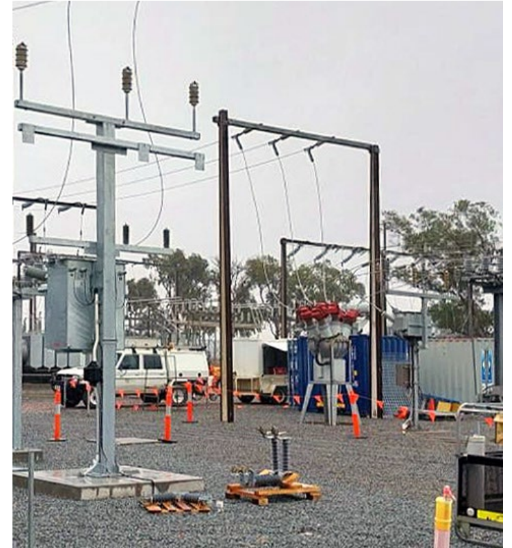
Upgraded Cleve Substation
