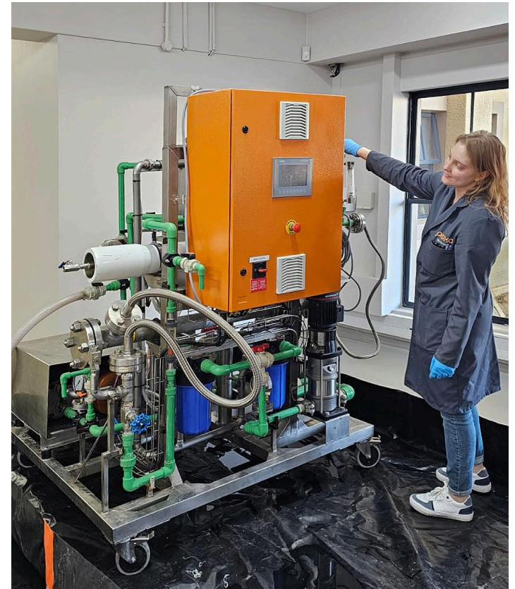
Waste-Water equipment trials, PSG Demonstration Facility
